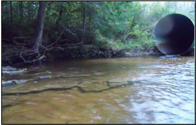
This downstream view of the culvert at Waveland Road shows the fish passage barrier, one of two that will be remediated on Milligan Creek.
