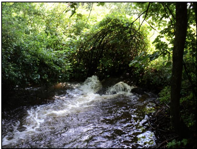
Improperly sized culverts such as this one on Sanborn Creek will be remediated to allow for fish passage.
